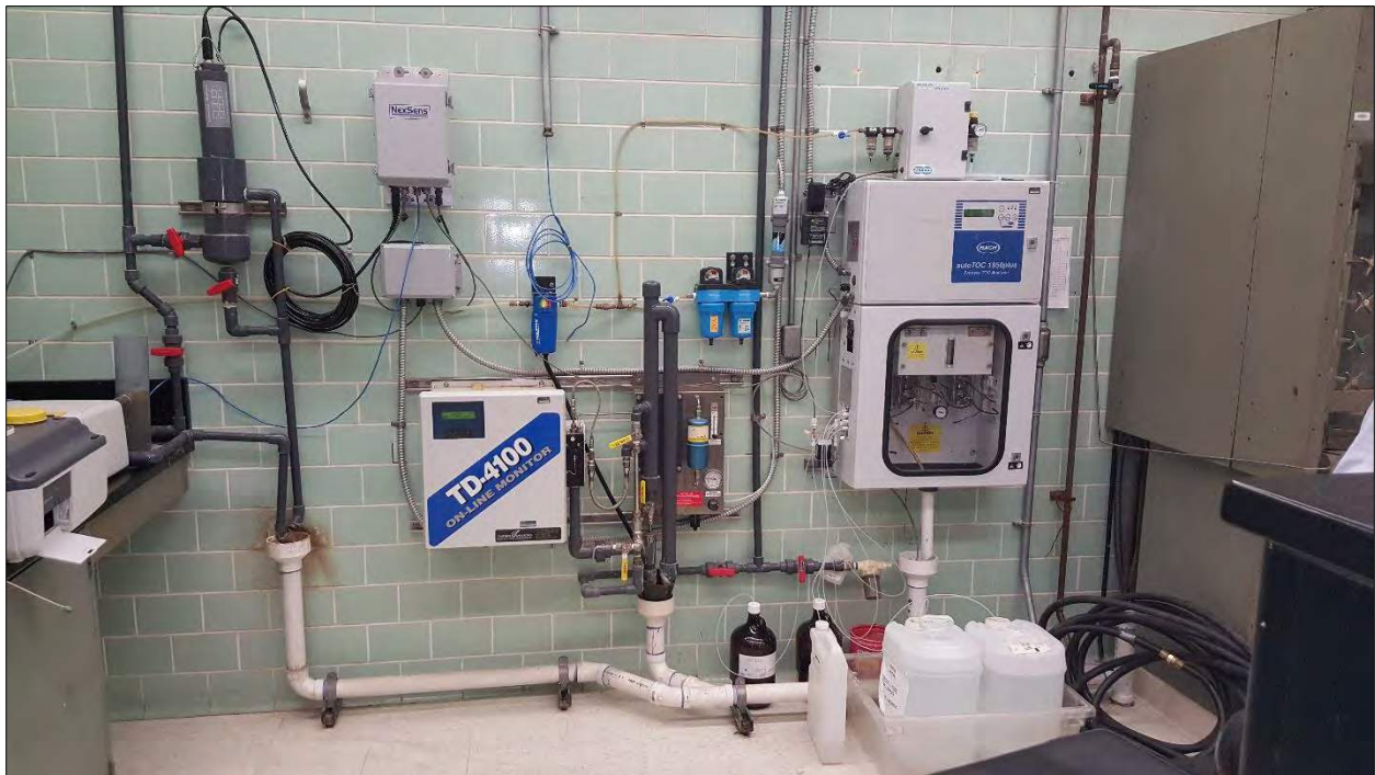
Figure 2: Drinking Water Monitoring Equipment – SW Detroit Water Treatment Plant (Complete site including Sonde, TOC Analyzer, Fluorometer, and GC-MS)
