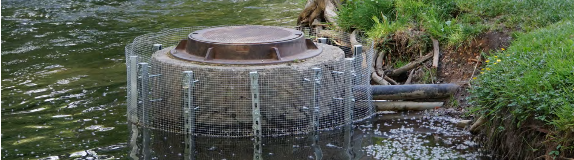
Sanitary sewer, Clinton River
