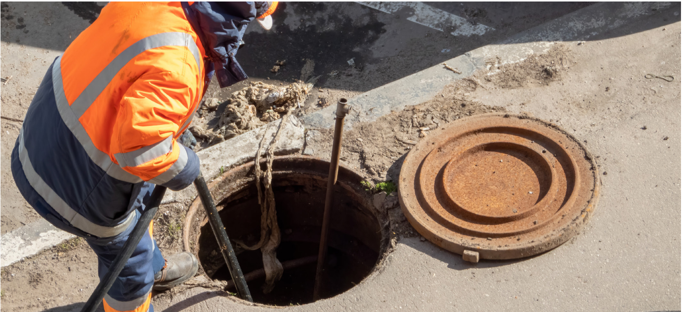
Figure 1. Routine stormwater infrastructure maintenance. Stormwater utilities commonly fund activities such as catch basin cleaning, storm sewer inspection, debris removal, and other operation and maintenance services needed to maintain drainage system performance and reduce flooding and pollution risks.
